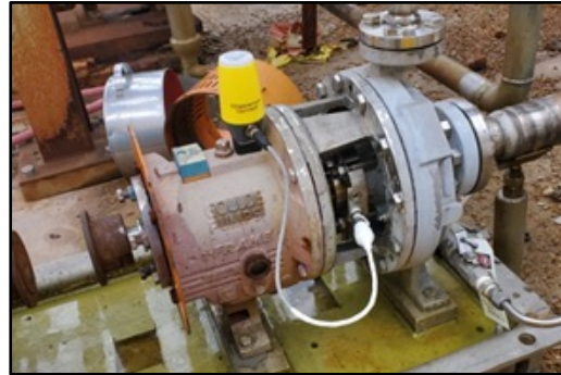
Chesterton Connect installed on the pump.
