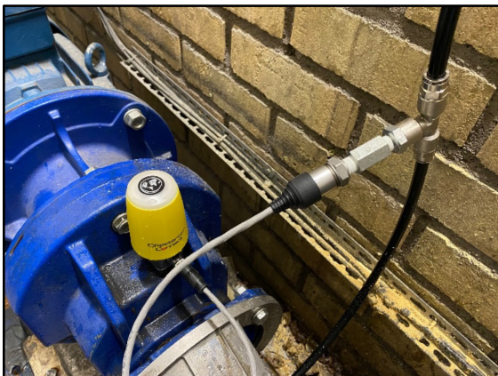
Chesterton Connect set to monitor barrier fluid.
