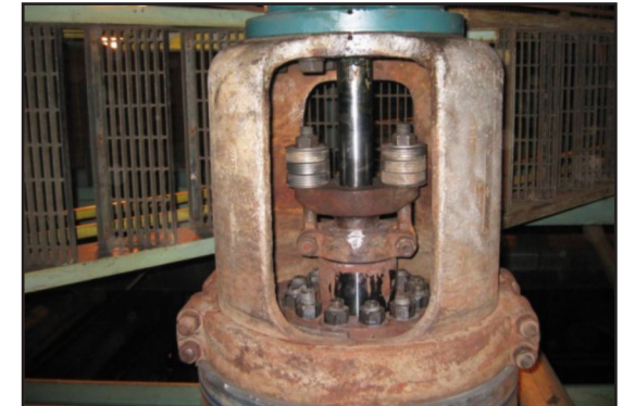
Critical plant valves have extended equipment life.
